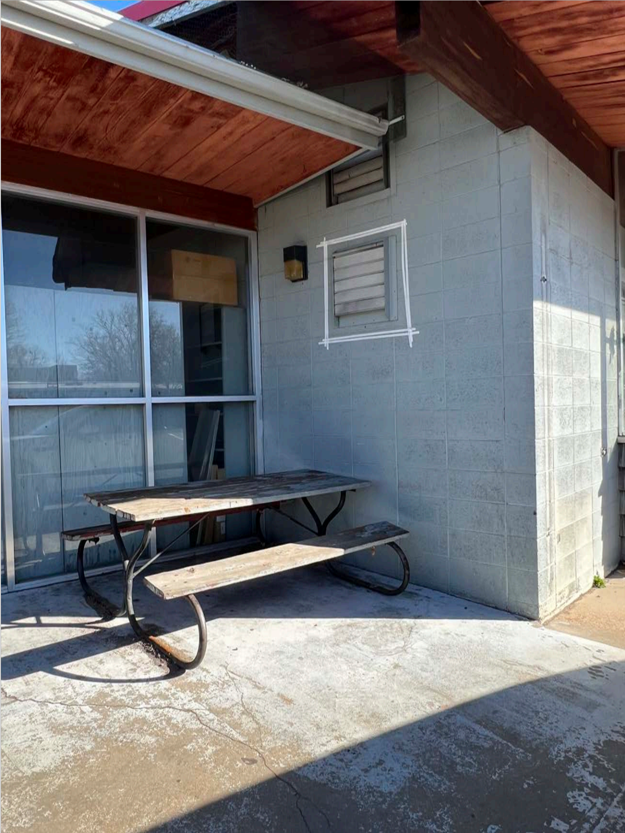
28. West Elevation - Back wall of the Showroom, south portion, detail. Image courtesy of BEE. 2024.
