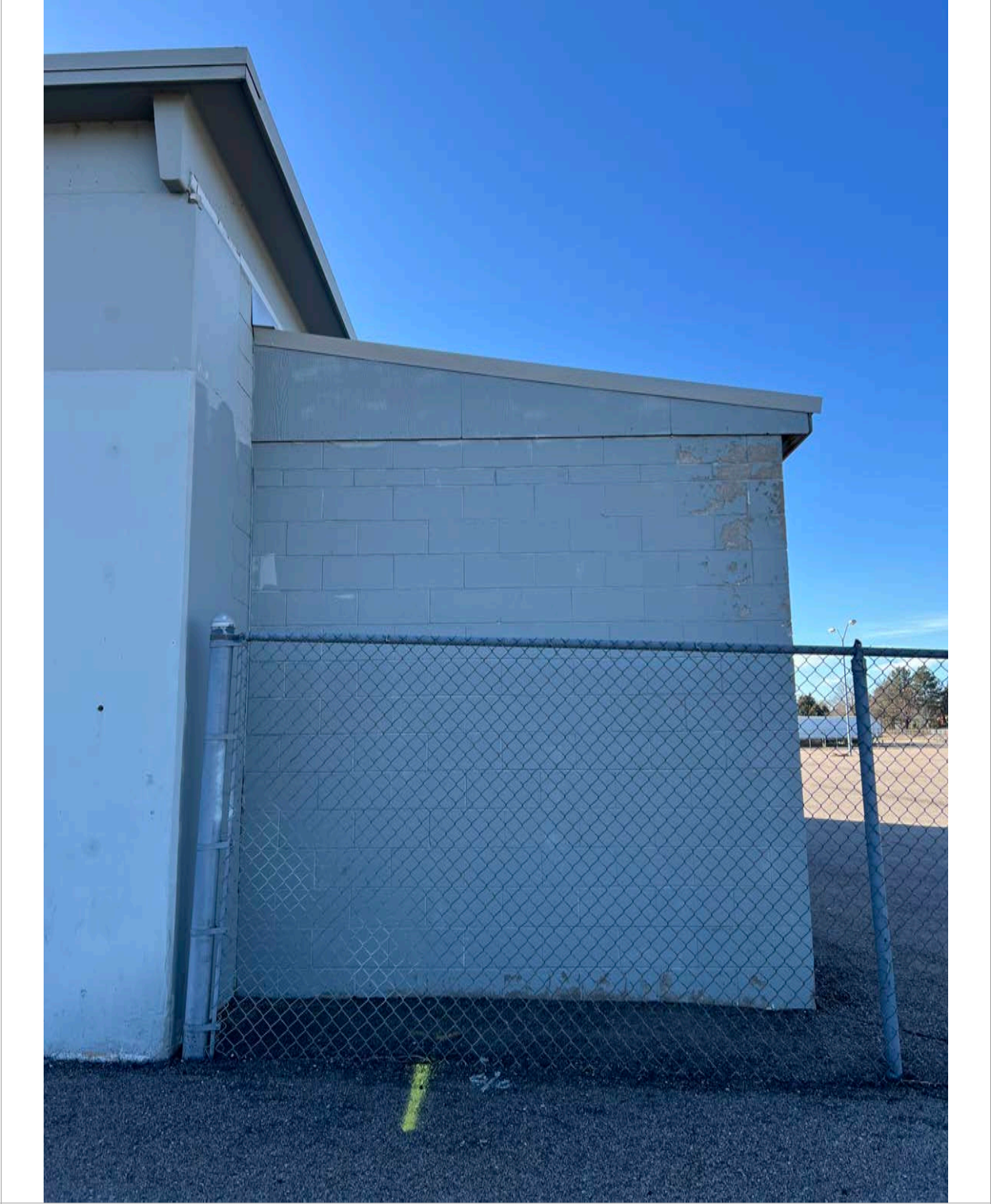
21. North Elevation - Shed addition at the back of the service center.. Image courtesy of BEE. 2024.
