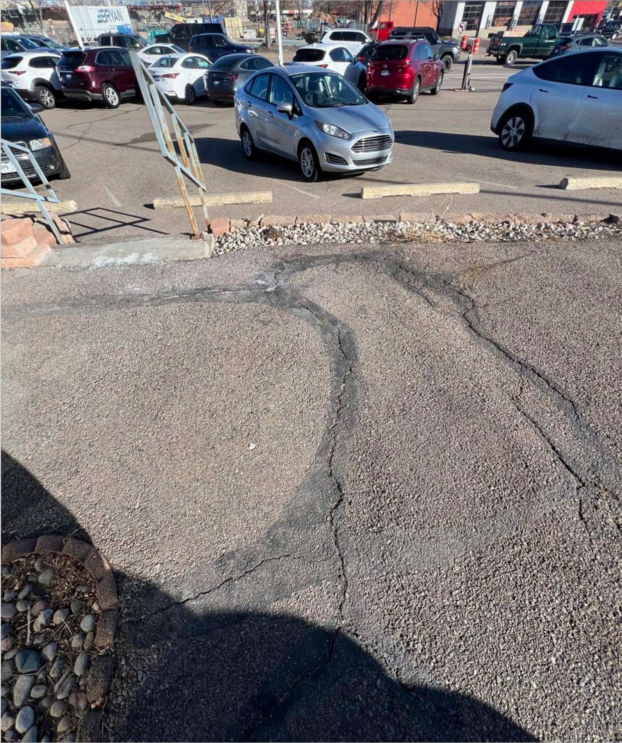
54. Site - Detail of deterioration on east side of Building B. Image courtesy of BEE. 2024.
