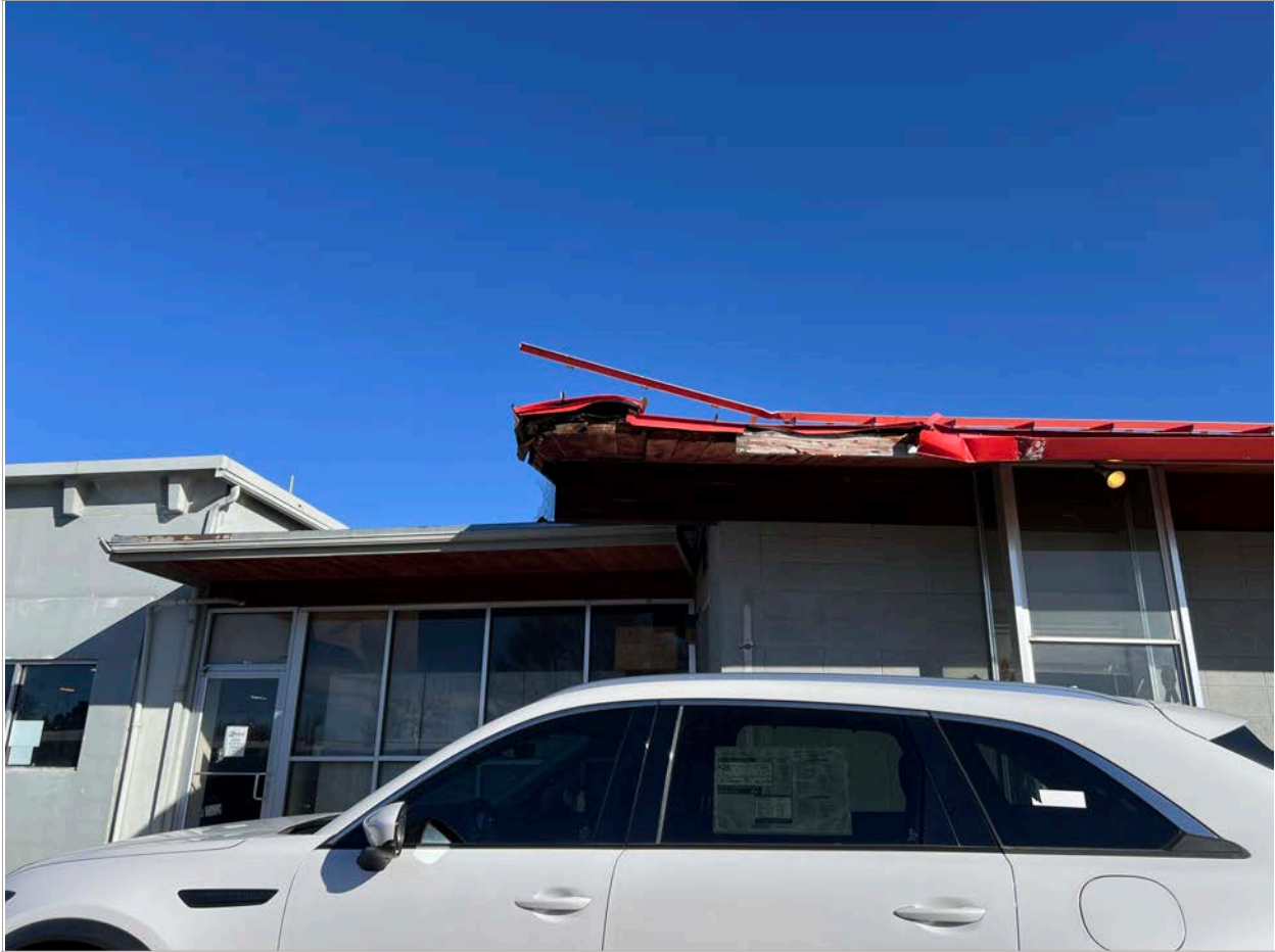
41. South Elevation - Detail of damage at roofline. Image courtesy of BEE. 2024.
