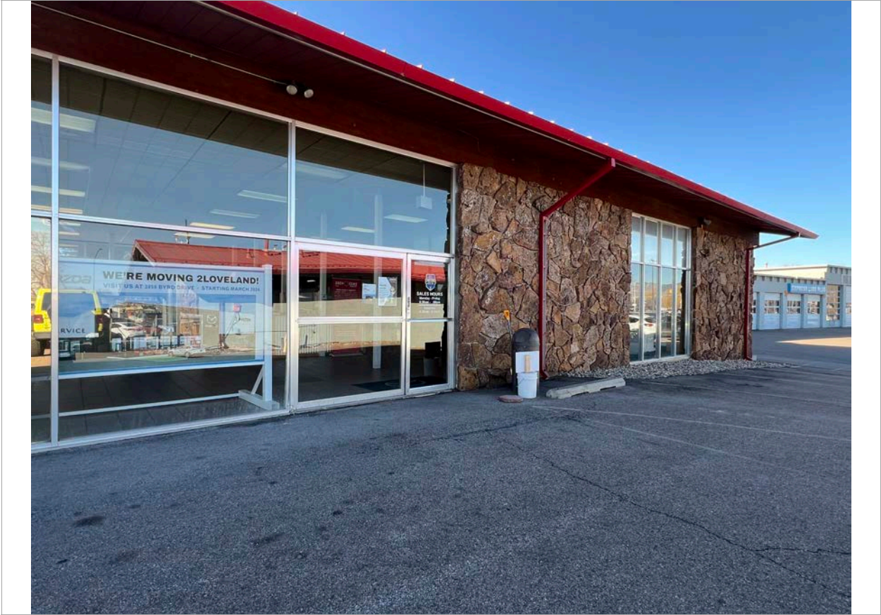
12. North Elevation - of showroom. Note door with hinged window to allow cars into the showroom, located in the middle of the photo frame. Image courtesy of BEE. 2024.
