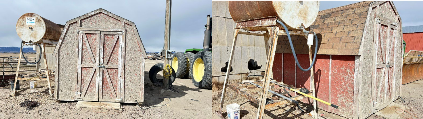
Building ID 507 Tool shed, wood frame, built in 1970, low quality, 168 sf Age: 54 years
