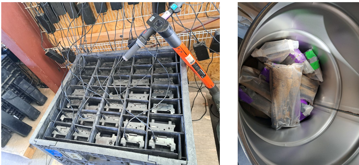
Figure 6. Batteries in the charging array (left) and packed in flame retardant for disposal (right)
