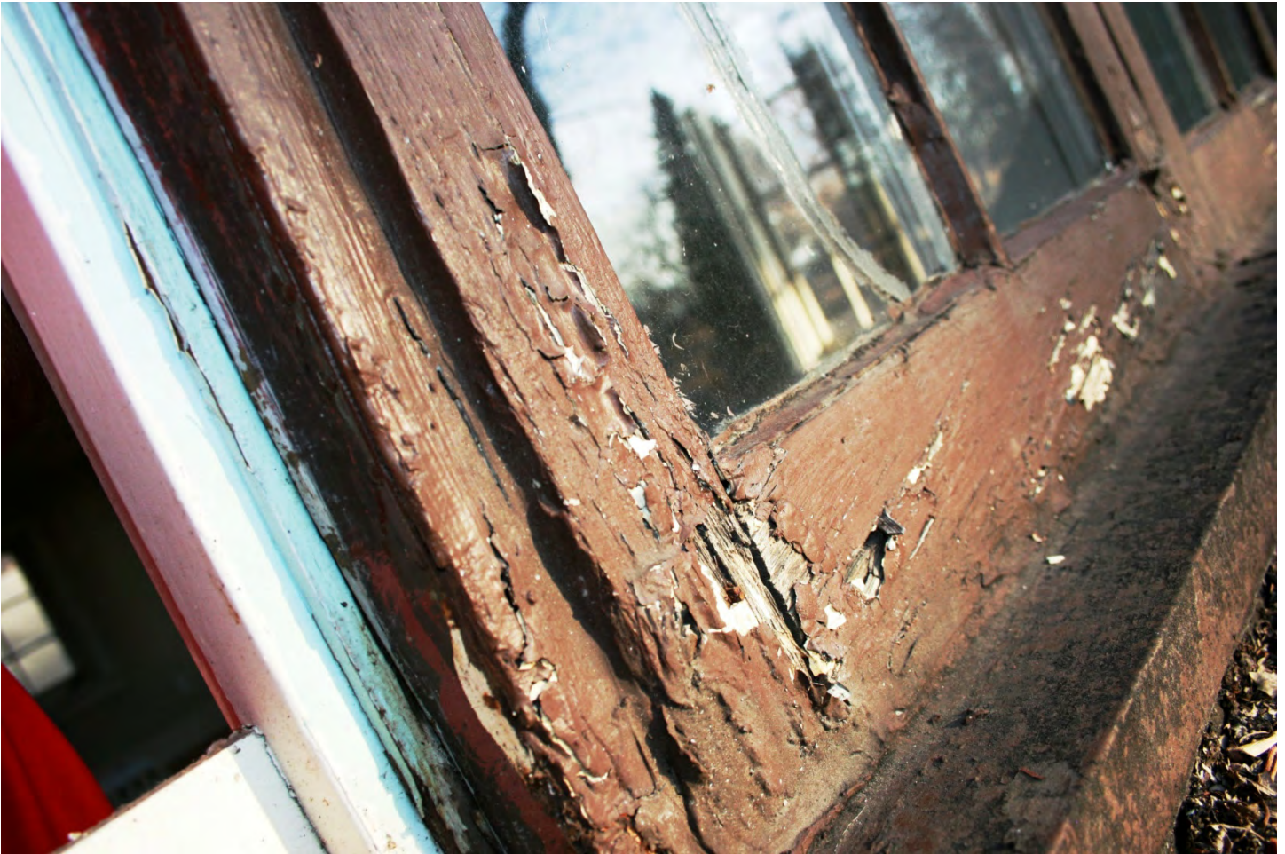
Image 5: Window 2-4. The lower rail, portions of both stiles, and portions of the muntins will likely require replacement
