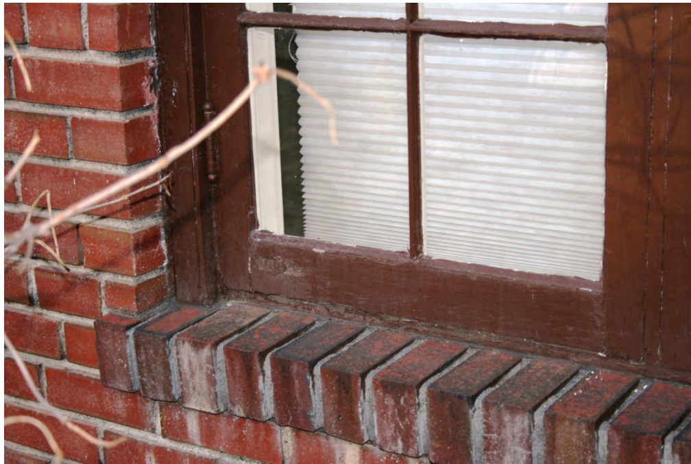
Image 3: Window 1-10, common exterior condition
