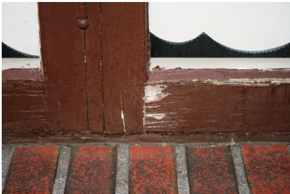
Image 4: Window 1-15, common exterior condition
