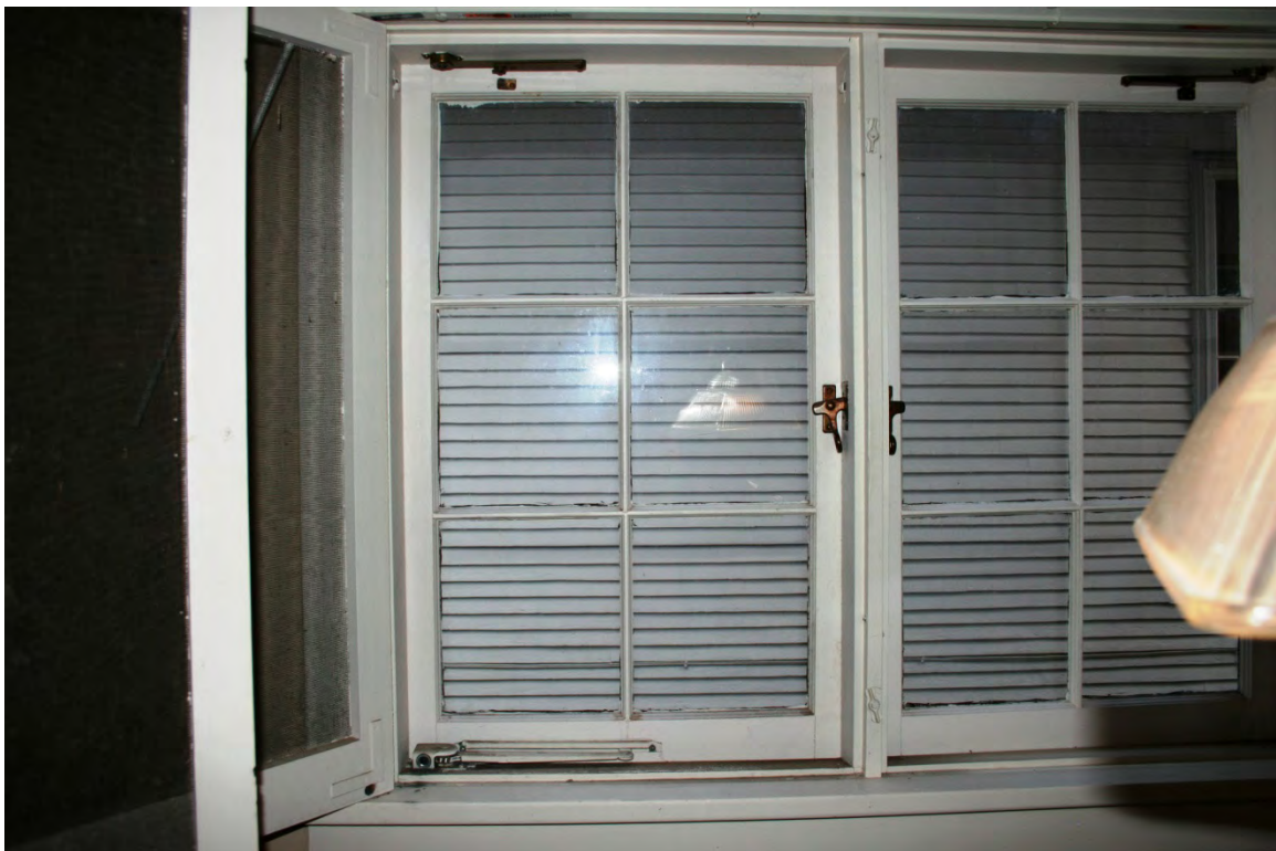
Image 7: This window has what appears to be the original hinging hardware at the head of the jamb.
