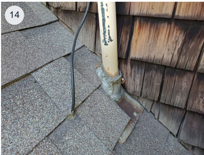
Metal pipe boot failing, water or electrical line through shingle and caulked.
