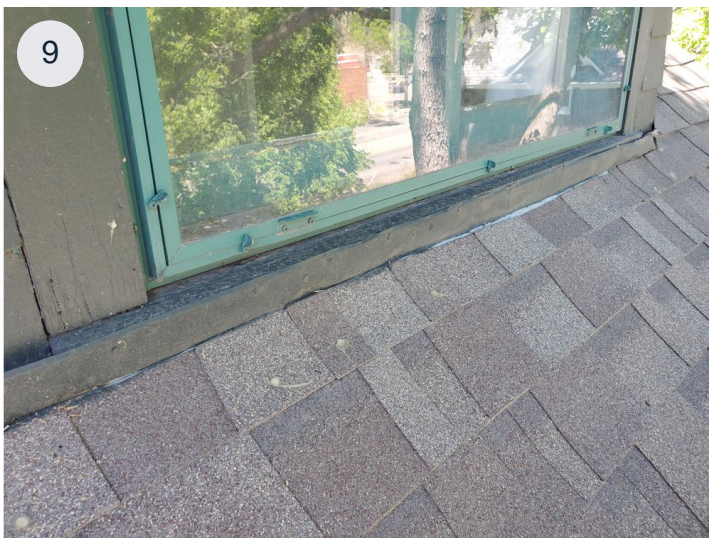
Window transition missing appropriate flashing
