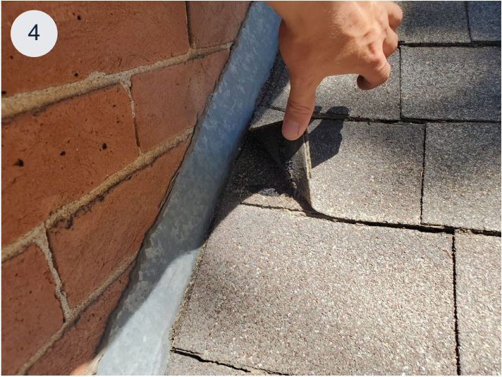
4 Shingles missing step flashing along all vertical running walls.
