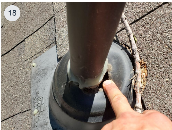
3" pipe boot old and failing, repairs not possible Recommend replacement
