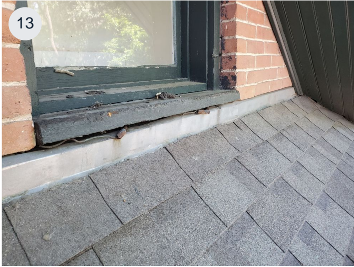
Window flashed improperly, missing counter flashing
