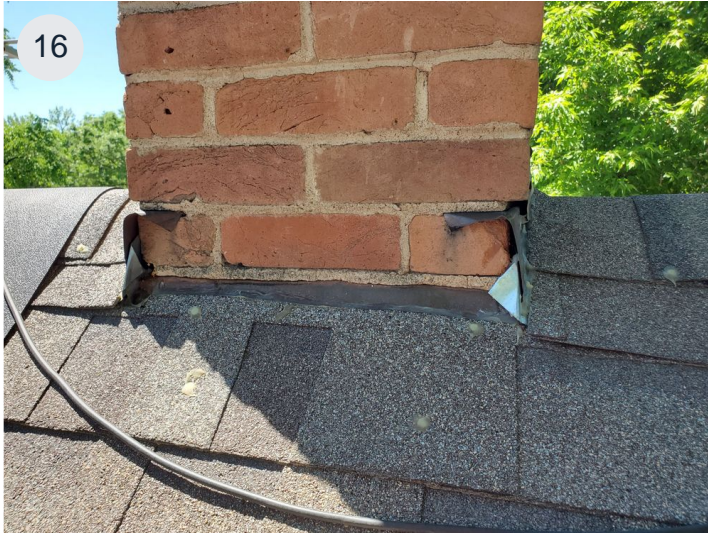
Chimney missing all appropriate counter flashing and front and back pans
