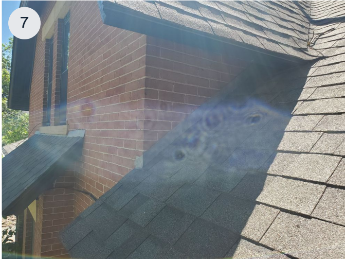
Missing step flashing and counter flashing
