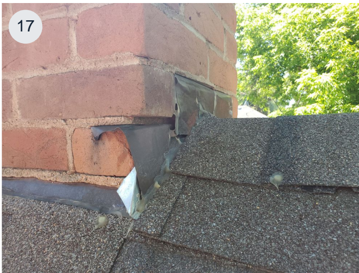
Missing step flashing and counter flash
