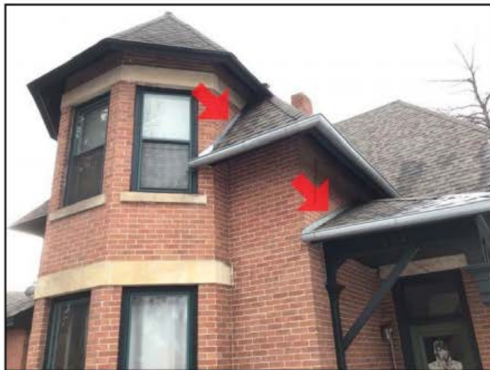
5. Not let into mortar joints
