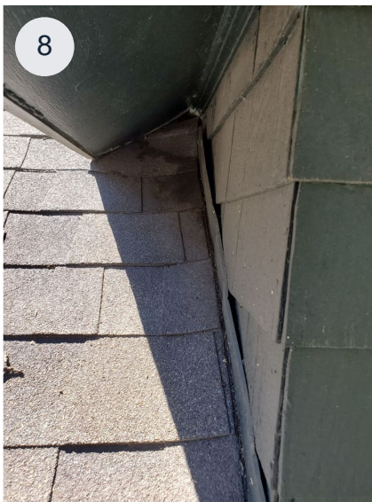
No step flashing behind siding, wall is flashed wrong allowing water to enter behind metal.
