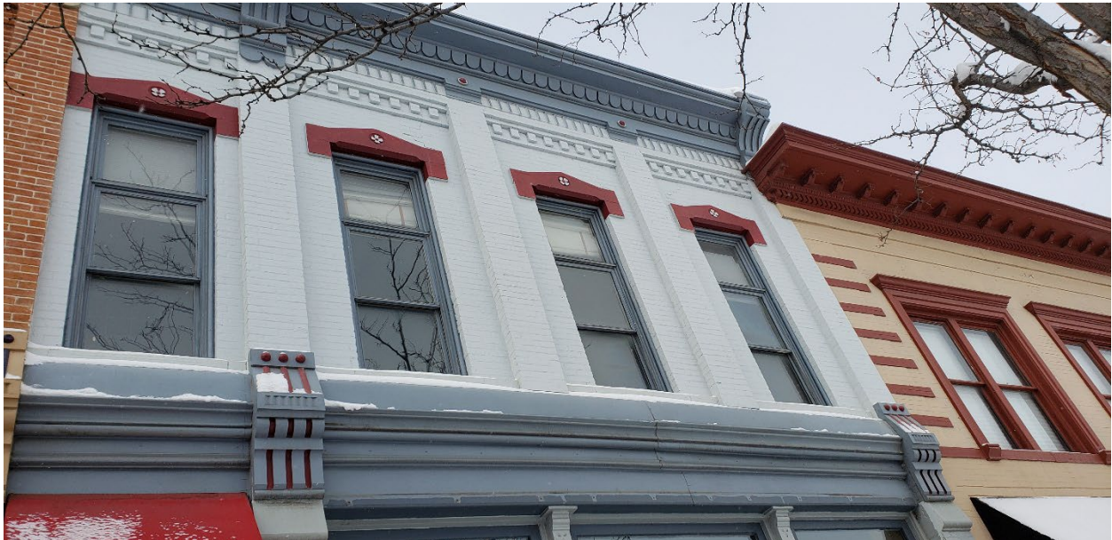
255 Linden/Standard Block – upper windows proposed for replacement.
