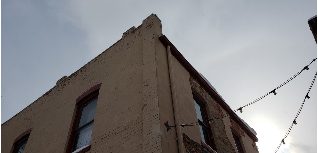
North corner of 261 Jefferson at upper story, showing masonry deterioration and sandstone cap.
