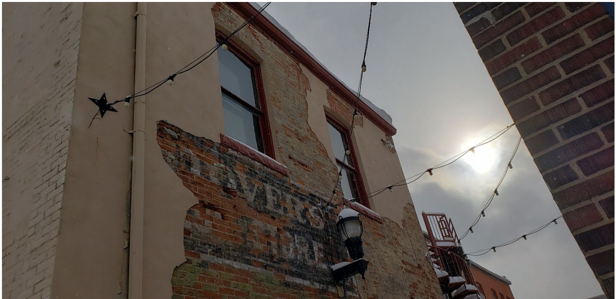
Northwest/alley side of 261 Jefferson upper story, showing masonry condition and ghost sign.
