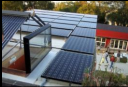
A. Rooftop solar panels
