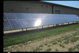
C. Ground solar array
